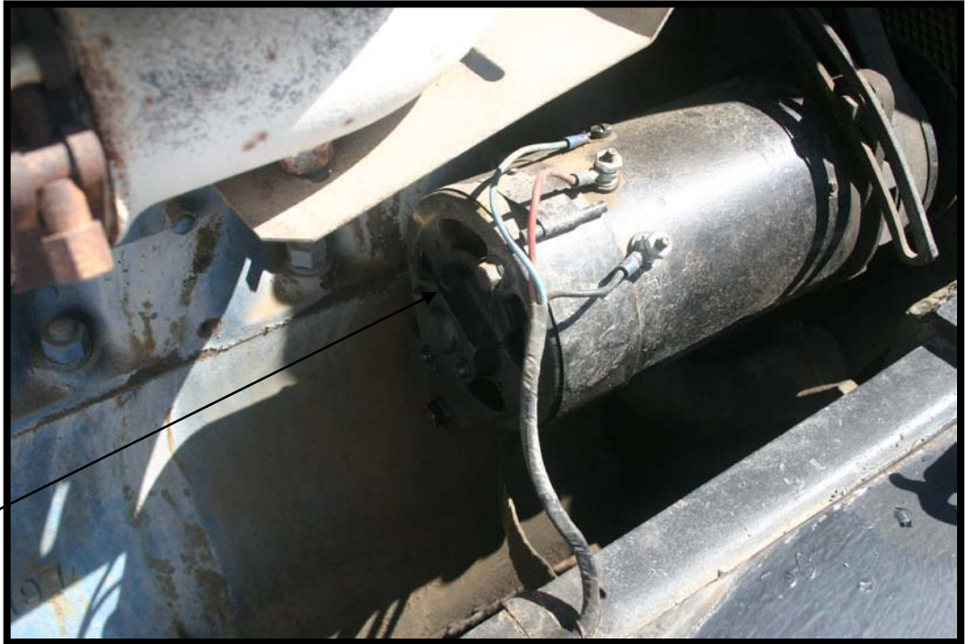
Generator, two oil cups.
